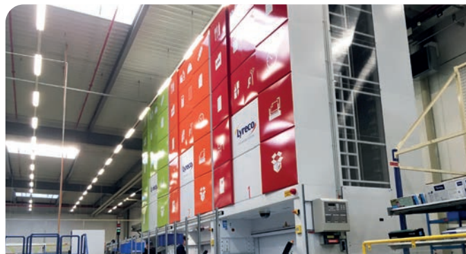
Fire protection system integration
